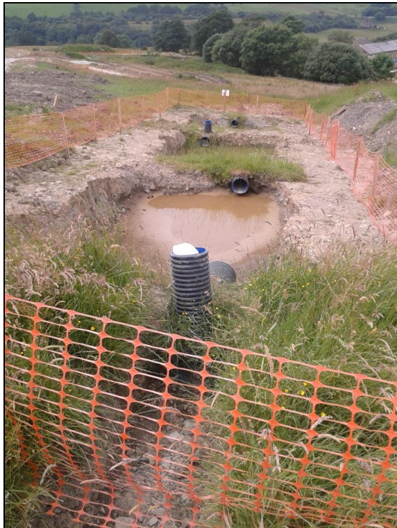
Plate 5: Typical lagoon and flocculent station
